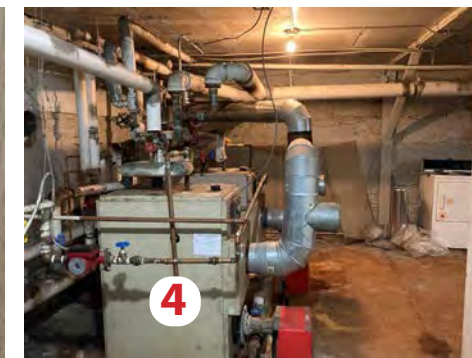
Furnace room in basement
