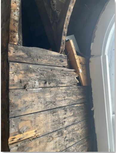
EXISTING ROT AND BANDAID MODIFICATIONS IN THE 80'S/90'S
