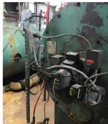
Figure 1 boilers at 245 Freshwater.
