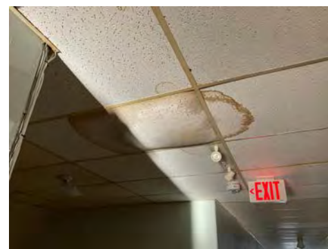
Fairly isolated occurrence of water damage
