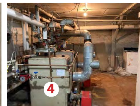
Furnace room in basement
